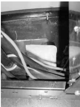
Figure 2. Place masking tape over the lamp sockets to keep metal shavings out of them.
